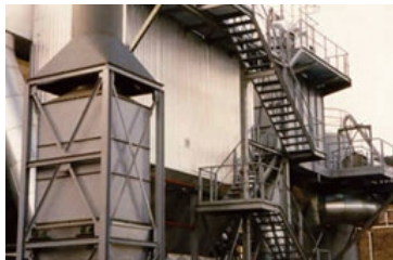
Aluminium Industry Dust removal after the furnace
