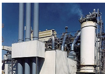
Cement Industry Dust Removal after lime-burning
