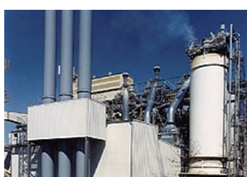
Cement Industry Dust Removal after lime-burning
