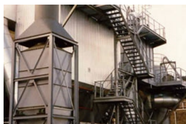
Aluminium Industry Dust removal after the furnace
